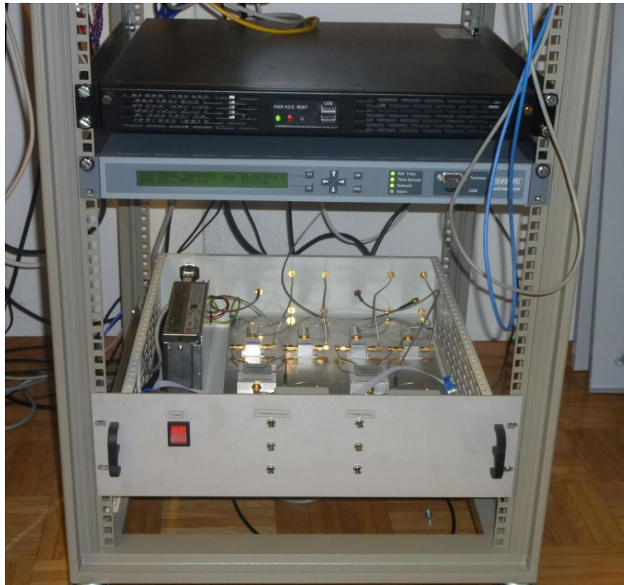
Downconverter, Data Grabber, System Control
